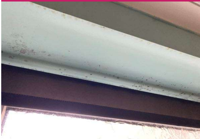
21-11-2022 12:38 / Bathroom Windows Sills / Rpjn3k0ry
