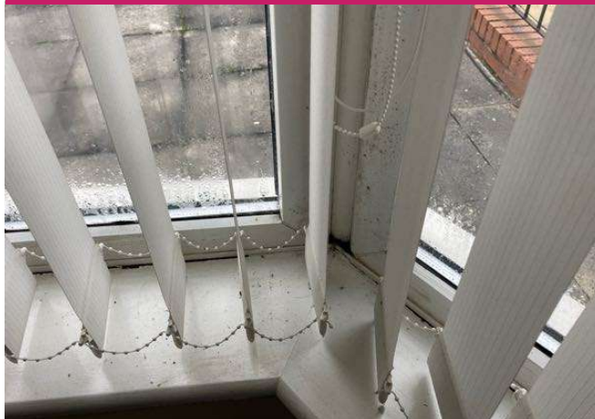
21-11-2022 12:35 / Windows Sills / Shxjiuw11
